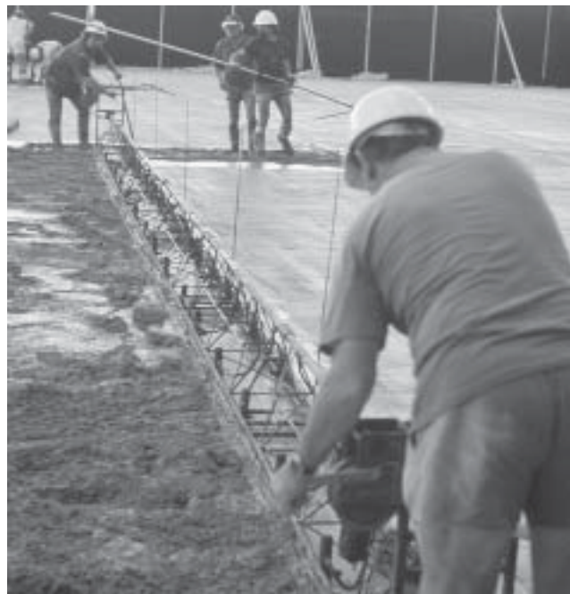
Slab being compacted with a double vibrating beam (note that the height of concrete is no more than 50mm above finished level)
